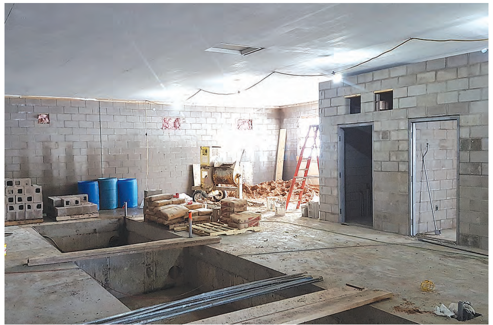
Pictou's new water treatment facility is currently under construction, but expected to be finished by Sept. 1.
