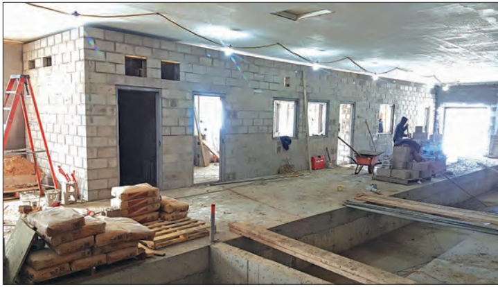
The new water treatment facility will include pressure zones to produce good water pressure throughout the town's higher and lower elevations.
