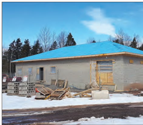
The exterior of Pictou's new water treatment plant is mostly complete while work continues inside.
